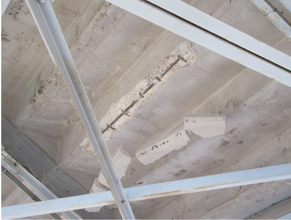
Figure 3. Concrete spall captured on netting.
