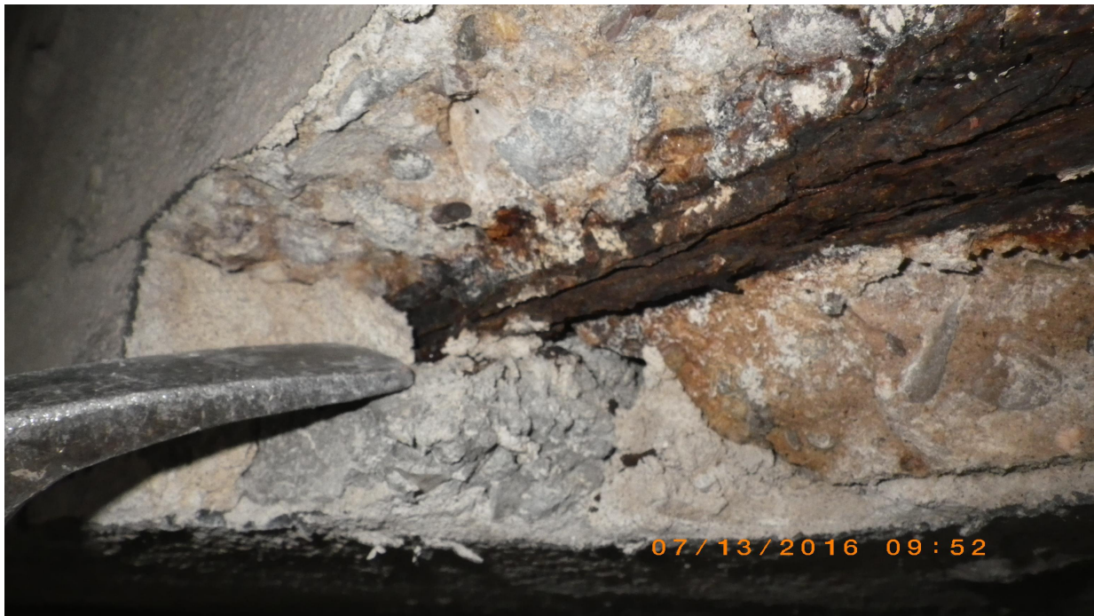
Figure 4. Concrete spall at prior repair. Note presence of multiple repair materials and lack of reinforcing steel undercutting.
