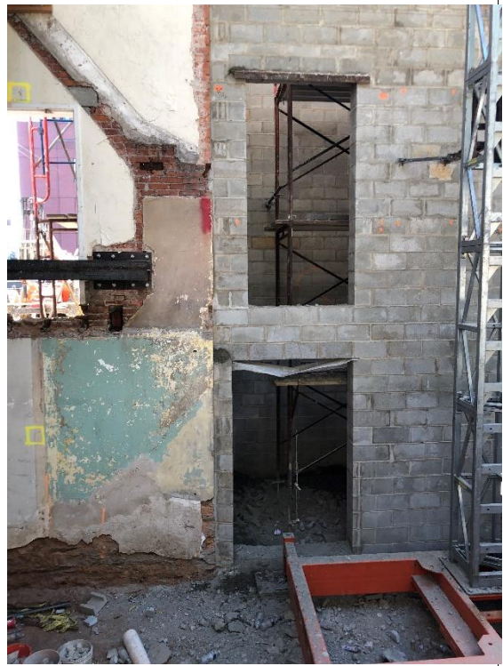
Above: Engineers knitted together the existing bearing wall and the new walls with anchors
