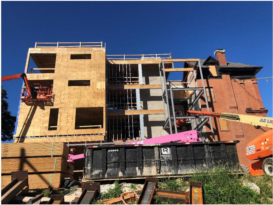
Above and Below: Overview of the building before the terracotta panels are added
