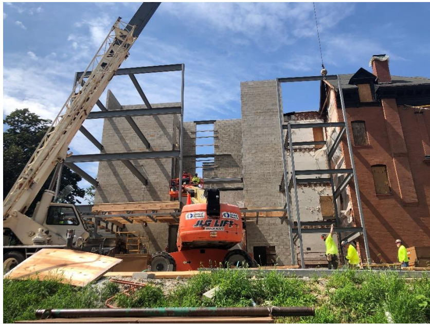
Left: Overall showing the multiple building systems, the existing masonry, the new steel framing, the CMU elevator shaft and stair tower, as well as the wood floor infills being installed.
