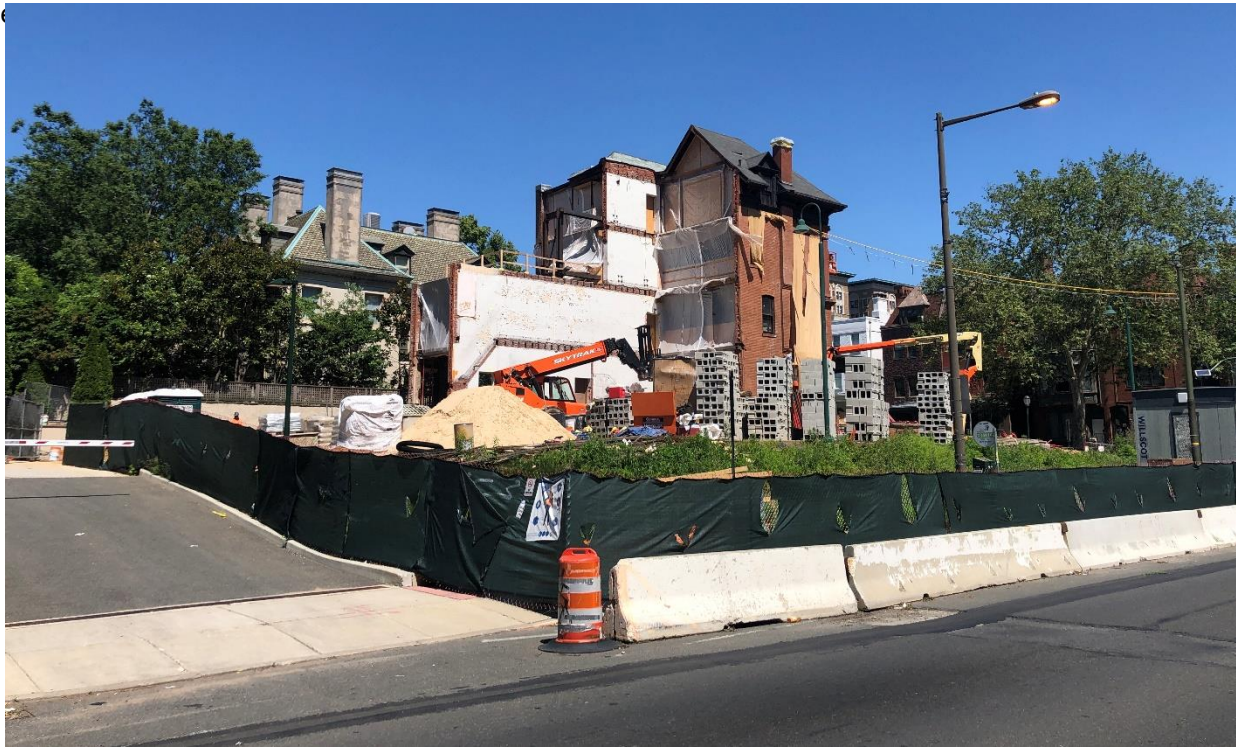
The design called for a large portion of the existing building to be retained. Selective demolition left the brick bearing wall which engineers had to knit the new steel framing and CMU stair tower into.
