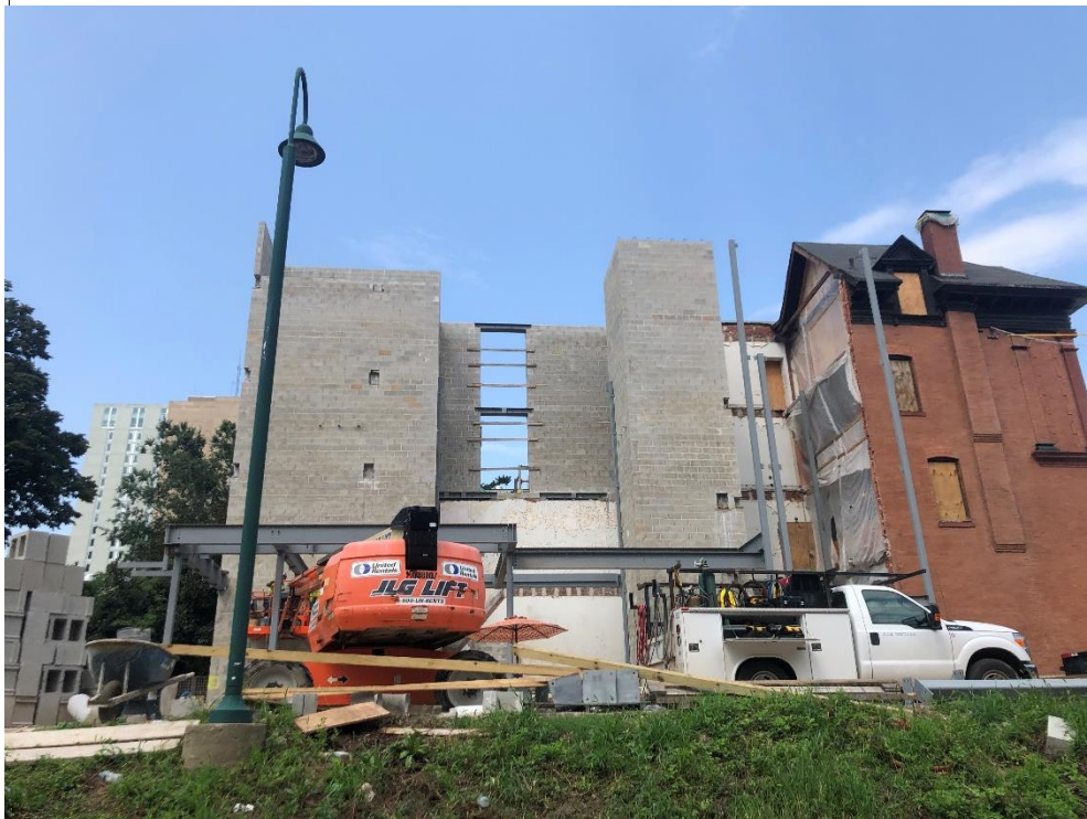
Left: Integration of the masonry for both buildings. Engineers reconstructed the shear walls using the new east stair and elevator tower.
