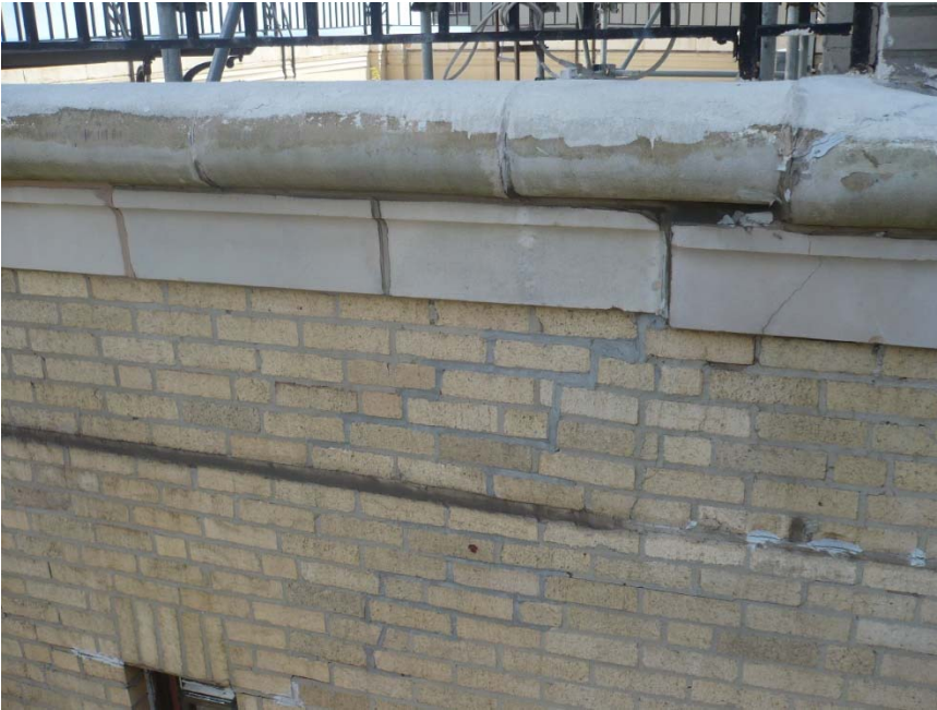
Figure 4: Caulk along spandrel beam mortar joint, brick and terra cotta cracking, parapet jacking.
