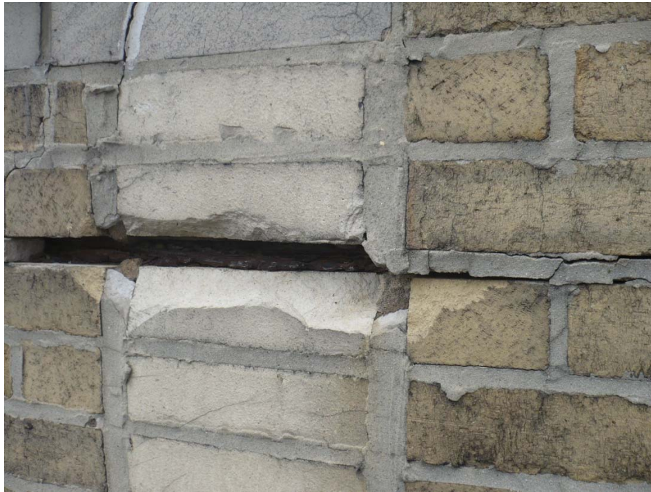
Figure 7: Corrosion jacking at spandrel joint and brick spalling.
