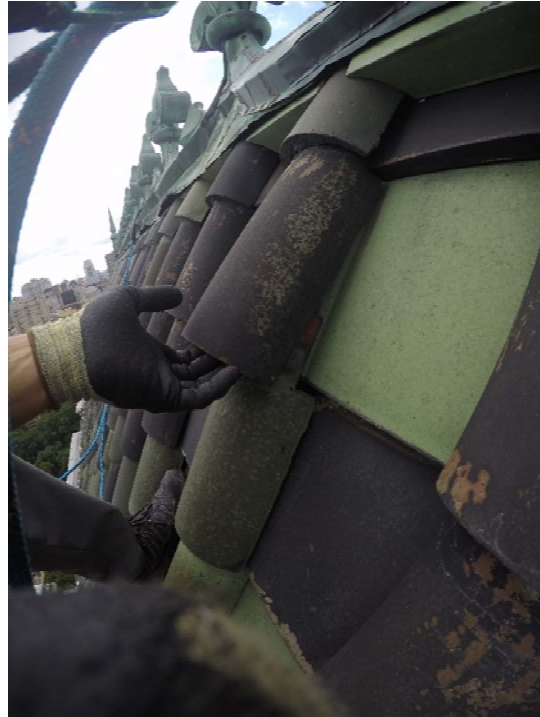
Figure 10: Detached roof tiles.
