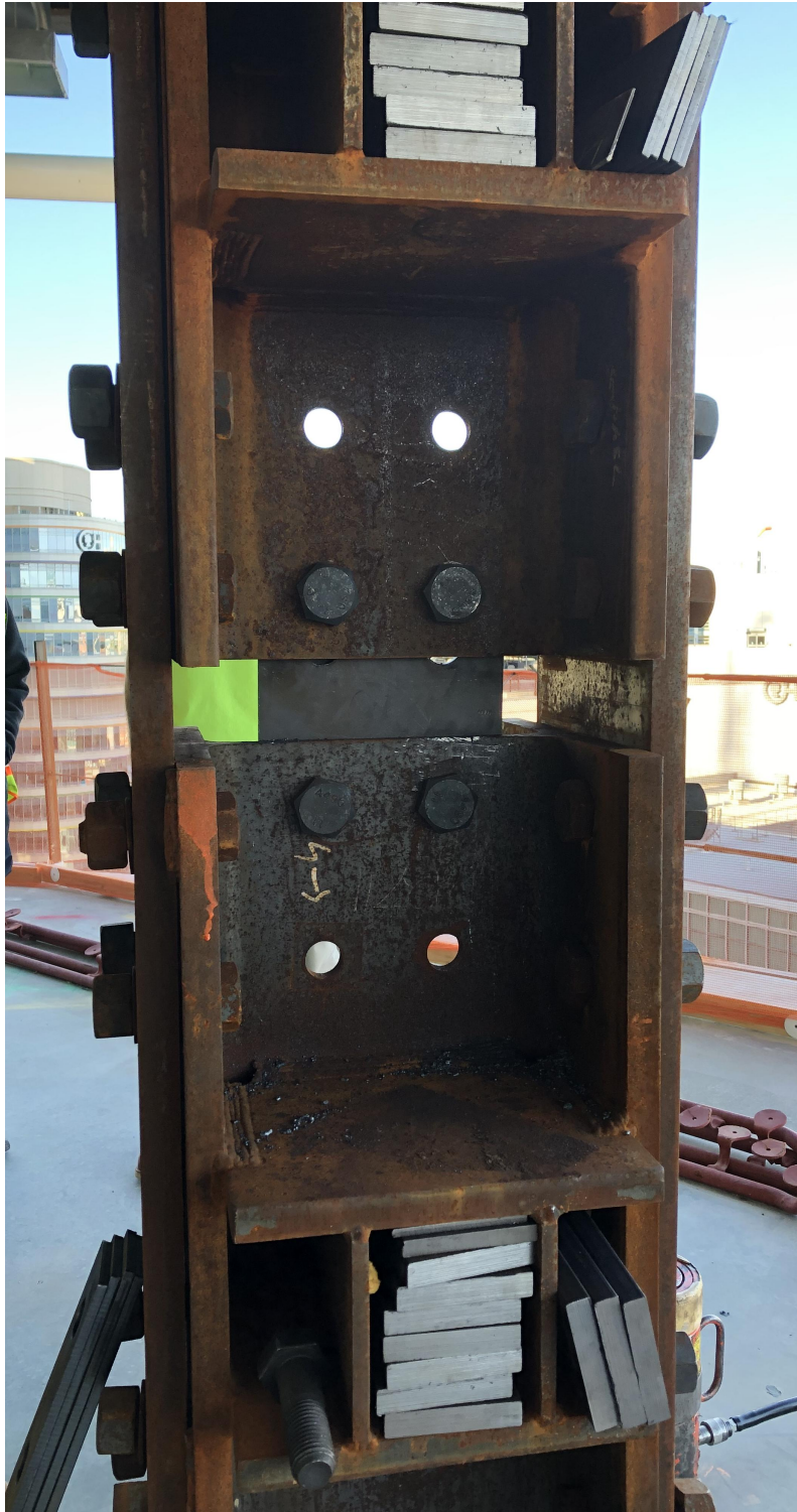
Penn Pavilion North End Level 9-10 Column Splice Detail - After Jacking with Shims Removed (Bolts Loose with Sustained Gap)
