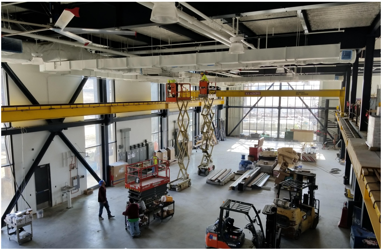
Above - The two story high-bay work space for CMU Robotics facility with the offset leg overhead crane. The crane rail to the left is higher for trucks backing into the building, while the rail on the right aligns with the second floor space.
